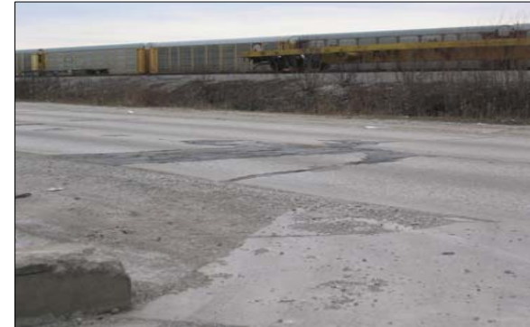
When the Village assumes responsibility for rights-of-way from other jurisdictions, it is presented with opportunities – and costs – to improve infrastructure conditions.
